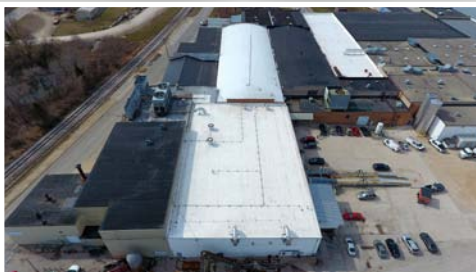
The last three years, a section has been reroofed at Lakeside Foods
